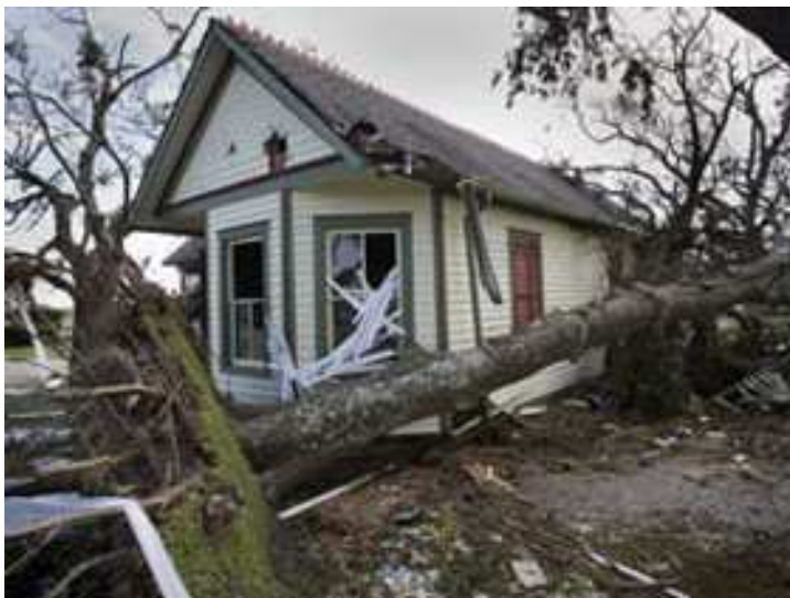
September 15, 2008, Wallisville, Texas. House destroyed by Hurricane Ike. Photographer: Gene Dailey/American Red Cross
